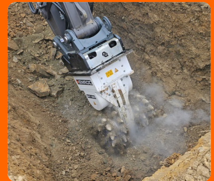
The rotary drum cutter attachment in action. Mounted on the large excavator, this attachment cut a large proportion of the solid dolomite rock.
