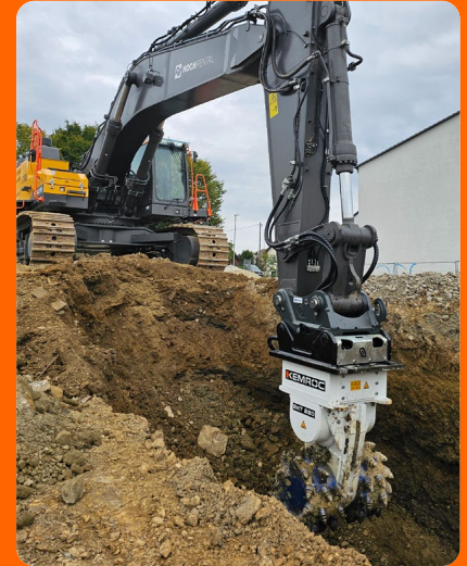
In consultation with KEMROC's sales consultant, the 75-tonne excavator was equipped with a KEMROC EKT 220 rotary drum cutter attachment.
