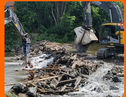
A second, smaller excavator plus hammer and bucket, broke out the individual concrete segments and transported them to the riverbank.
